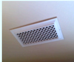
Installed without caulking
